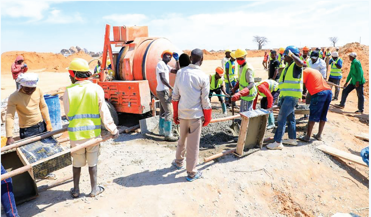
Men at Work: The ongoing construction of ITRACOM Fertilizer Limited factory at Nala Industrial area in Dodoma.
