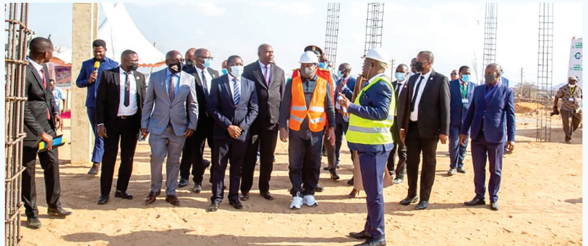
Burundi President His Excellency Evariste Ndayishimiye inspects the ongoing construction of ITRACOM Fertilizer Limited factory at Nala Industrial area in Dodoma during the official ceremony to inaugurate the factory in October, 2021.
